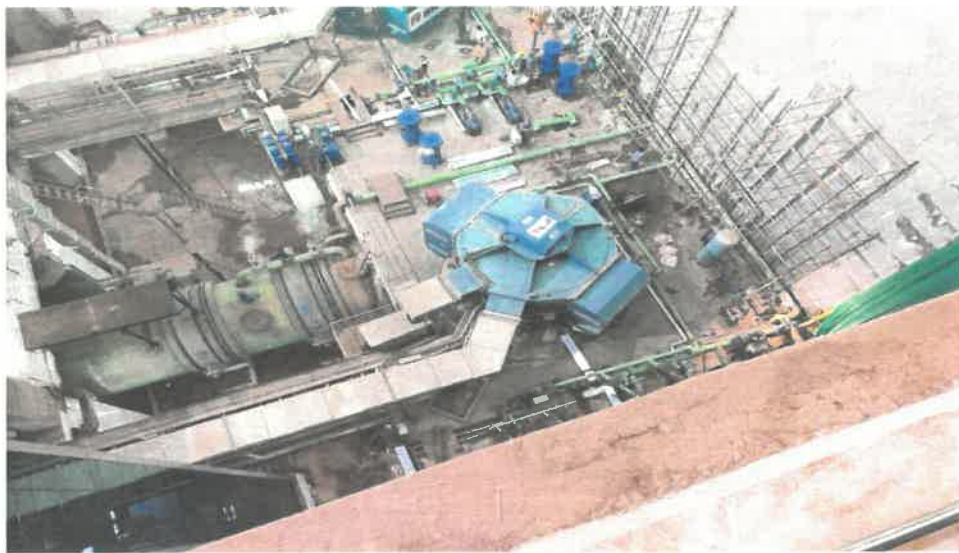
Pump House at Kaleshwaram Project
