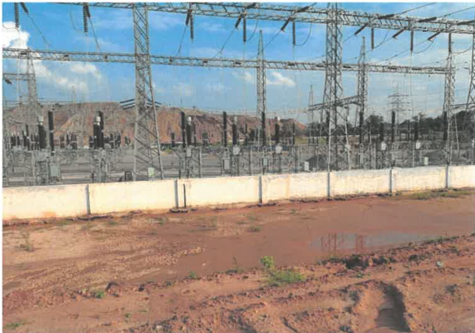
Power station at Kaleshwaram Project
