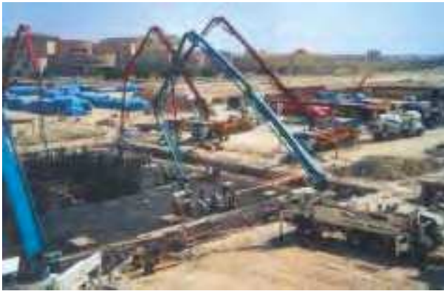
Concrete Pump and Placing Boom at Work in a Major Construction Site.
