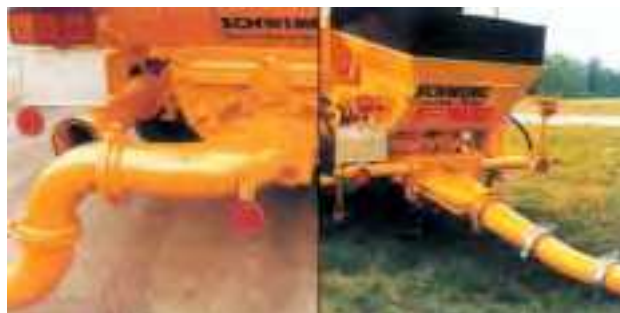
Pump and pipeline
