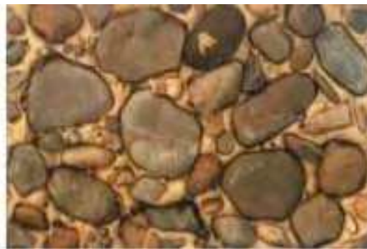
Badly pumpable concrete
