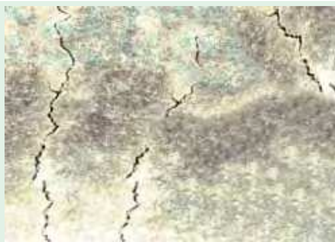
Fig.6.24. Cracks on concrete surface due to inadequate curing.
