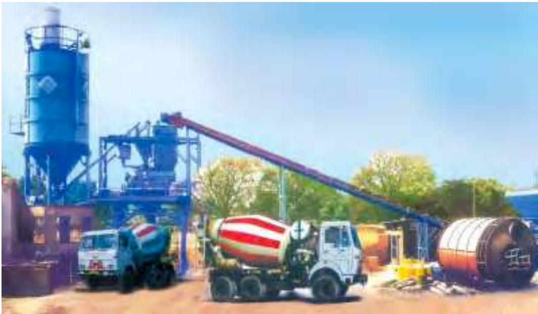
Modern ready mixed concrete plant.
