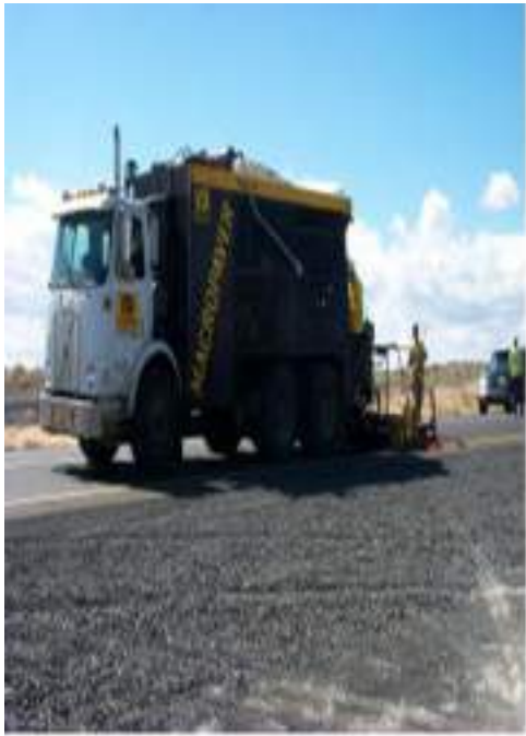
Figure 1: Ignition method major equipment.
