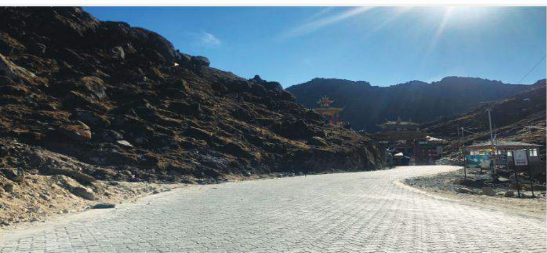
Paving of roads using M50 grade concrete blocks at Sela top (13680 ft).
