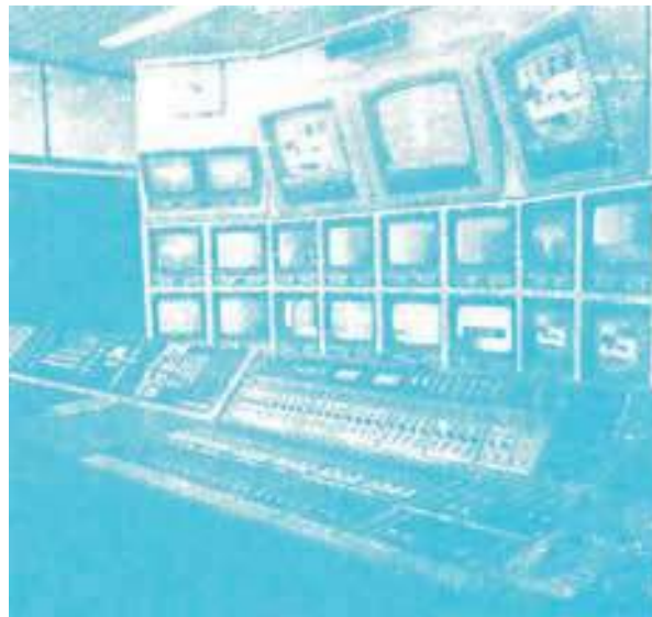
Fig. 7.3. A typical programme control room.
