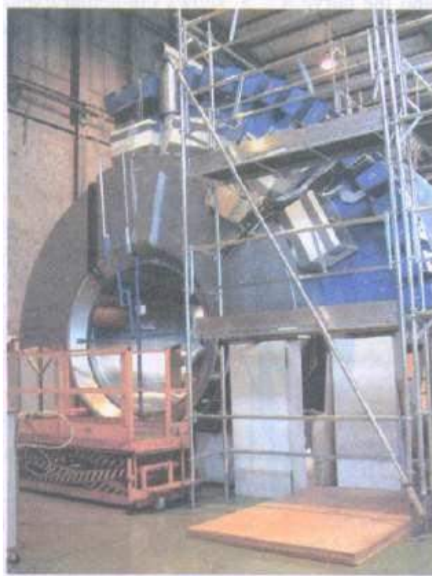
Air evaporative cooling system
